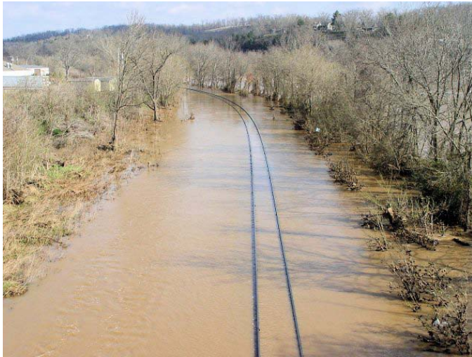
Figure 24. Flooded railroad along the Spring River in Arkansas
